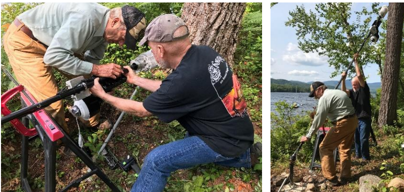
KLWA CCO volunteers installing the KLWA weather station on the east shore of Kezar Lake (south of Boulder Brook). Photo Credit: Don Griggs.
